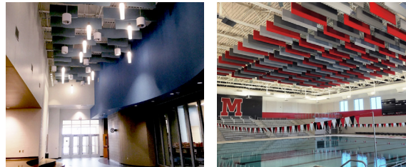
Left: Reedville Elementary School: WHISPERWAVE™ Baffles
