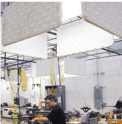
SONEX Valueline Baffles hung from ceiling mounts.
