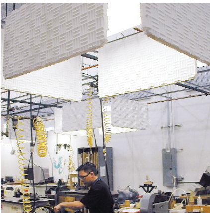
SONEX Valueline Baffles hung from ceiling mounts.
